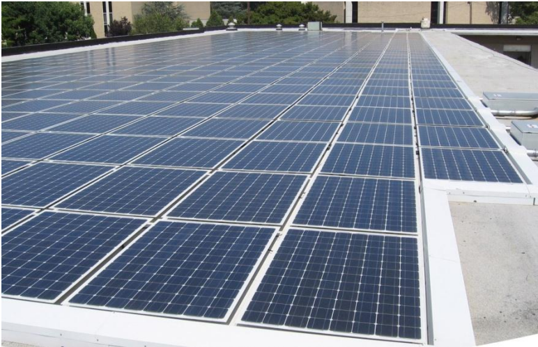
On-grid roof solar system
